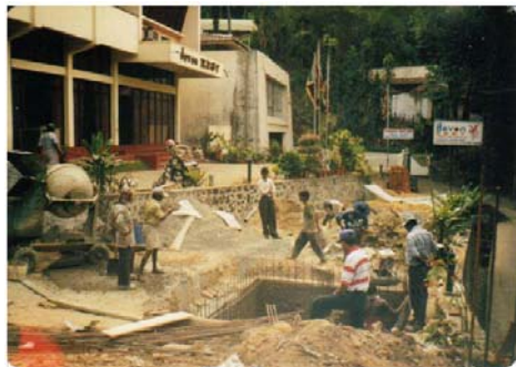
Figure 25: Entrance and driveway of the Devon Rest Hotel during construction of the anaerobic filter unit
