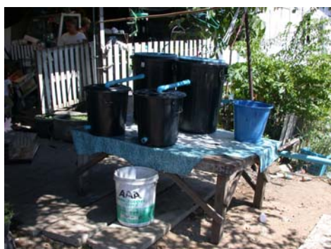
Figure 24: Two bucket greywater treatment system
