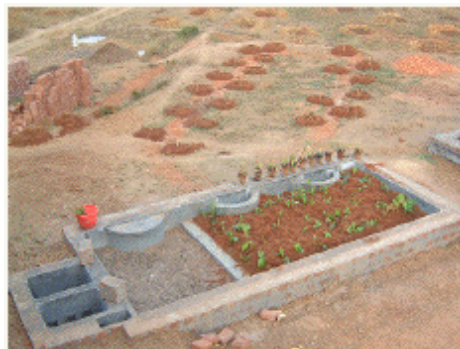
Figure 17: Greywater treatment system
