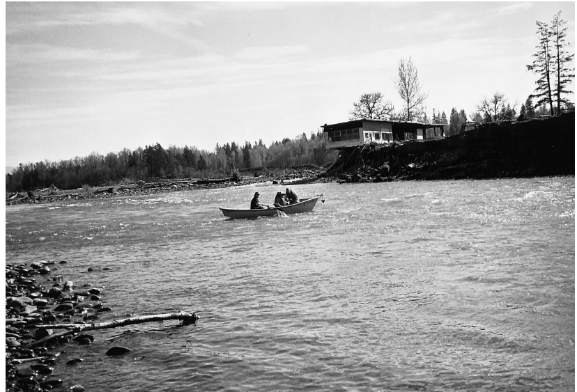
Figure 17. Building undercut by bank erosion as the Clackamas River flows through a captured gravel pit near Barton, Oregon. (Photograph by the author, April 1996.)
