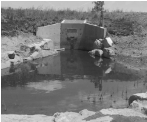
Figure 3. Micro-Pool and Outlet Structure Following Modification. Note 10-year rectangular overflow orifice above the water quality outlet (see Figure 2), and 100-year overflow with sloping rack on top of structure. Submerged bench and wetland planting aspect in the foreground. [Photograph used with permission of Urban Drainage and Flood Control District (UDFCD).]
