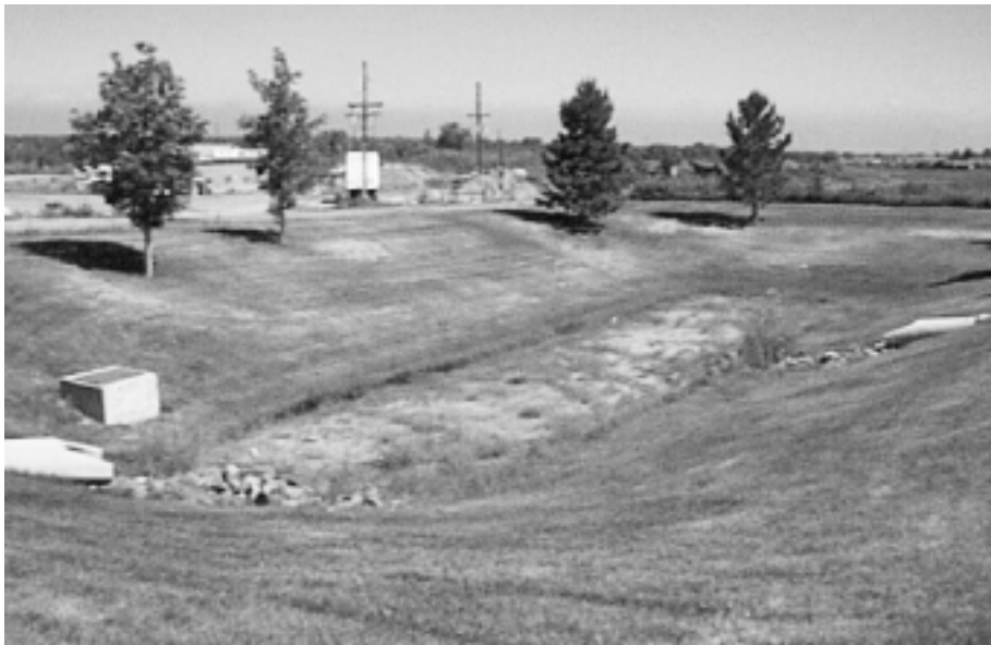
Figure 2. Sand Filter With Water Quality Capture Volume Above It, Installed in the Late 1980s. Note two inlet pipes and an overflow for larger storms.
