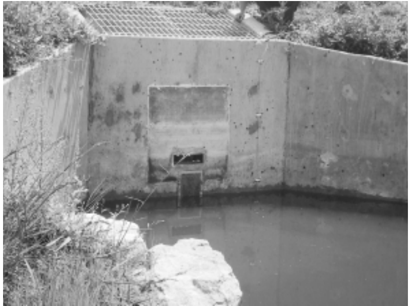
Figure 1. Extended Detention Outlet Installed in June 2001 and in Operation in August (18 hours after a storm's end). Note the partially submerged well-screen-type trash rack, the debris line that is near the bottom of the 10-year control orifice and the 100-year overflow on top. (This photograph was used by permission of the Urban District, Denver, Colorado.)
