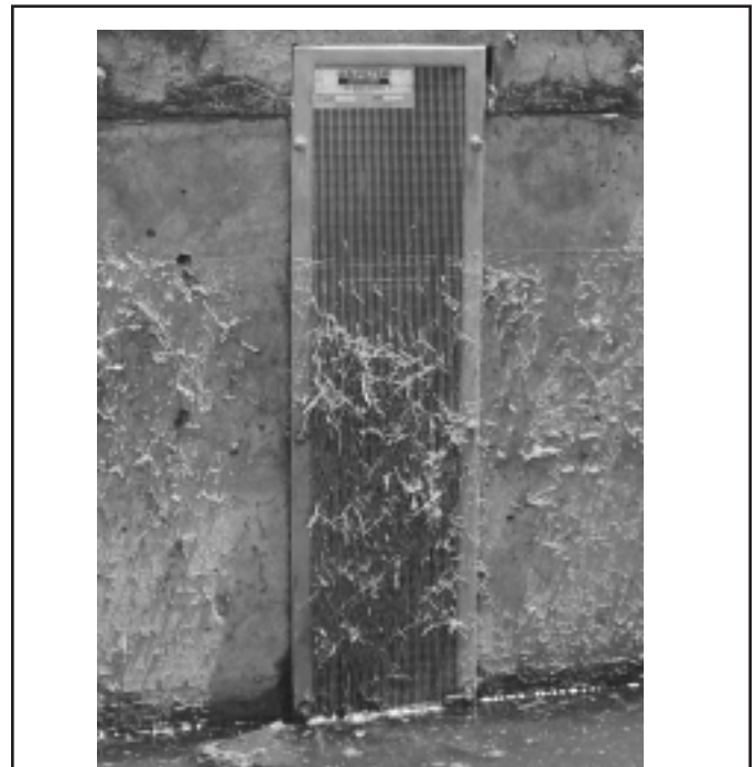
Figure 2. Close-Up of the Well-Screen Type Trash Rack. An orifice plate (not shown) is mounted on the inside of the concrete wall behind the trash rack. Note the high-water mark and the fact that grass clippings did not plug the trash rack. [Photograph used with permission of Urban Drainage and Flood Control District (UDFCD).]
