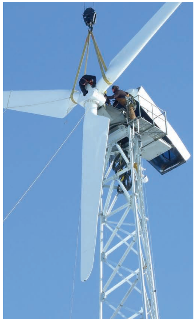
A Vestas V-15 rotor being installed on the turbine by a crew of four.
