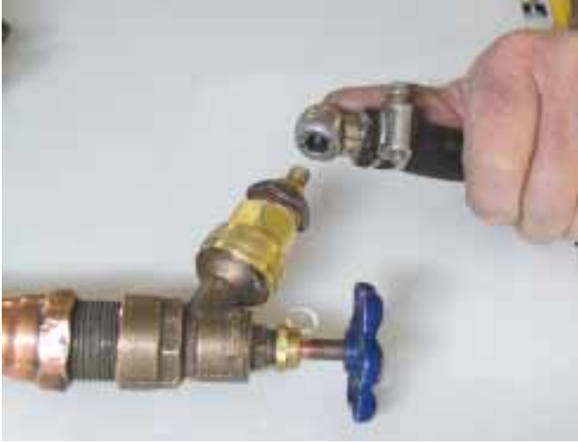
A pressure test fitting made from a Schrader valve and a female hose fitting.
