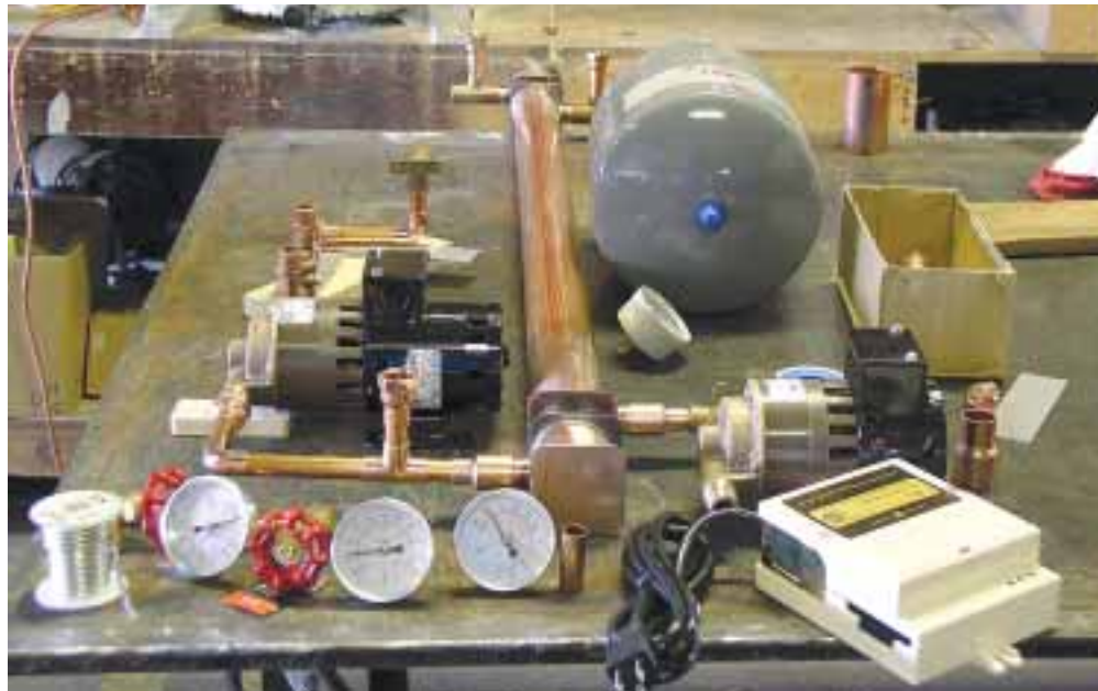
Laying out the components and plumbing parts in advance prevents headaches after the soldering begins.
