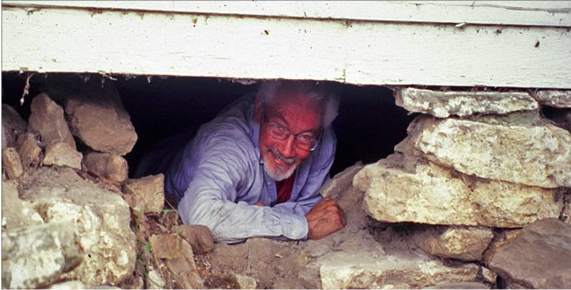
Fig. 3: The author emerging triumphant from an examination of the ground floor framing of the Mrs Sam Houston House in Independence, Texas. Field study is not always a clean activity, but it has no equal in developing respect for the structure and its makers, and in challenging the practitioner to use judgment as well as knowledge. Photograph by Samer Al Ratrout, 2003.
