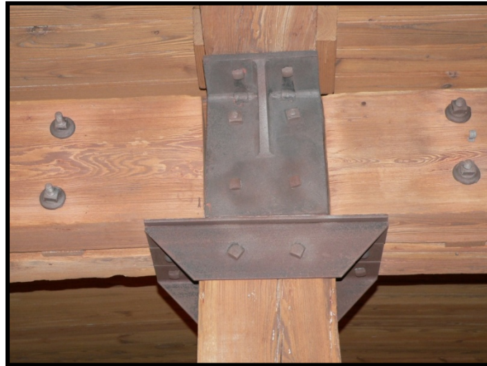
Beam-column connection with unknown capacity
