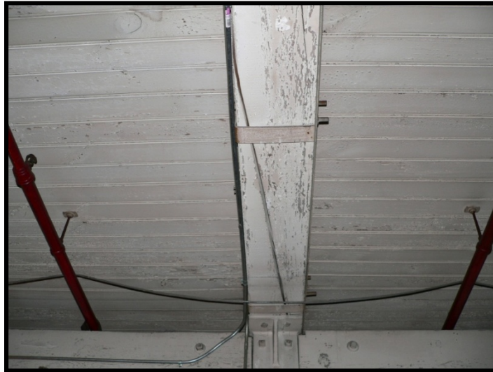
Makeshift structural repair using steel strap and plate
