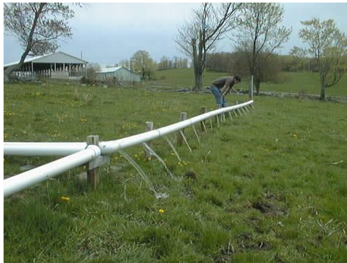
This perforated pipe allows a large volume of wash water to be discharged across a vegetative treatment area sufficient in size to absorb the discharged water before it can enter ground water or surface water. Photo: Joshua Faulker.
