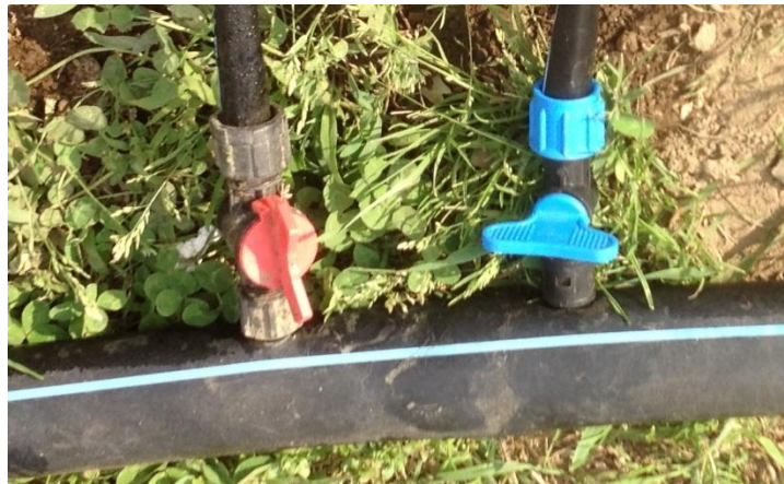
Valves can be added to drip lines coming off of the main line to allow irrigation to be turned on and off for individual rows.
