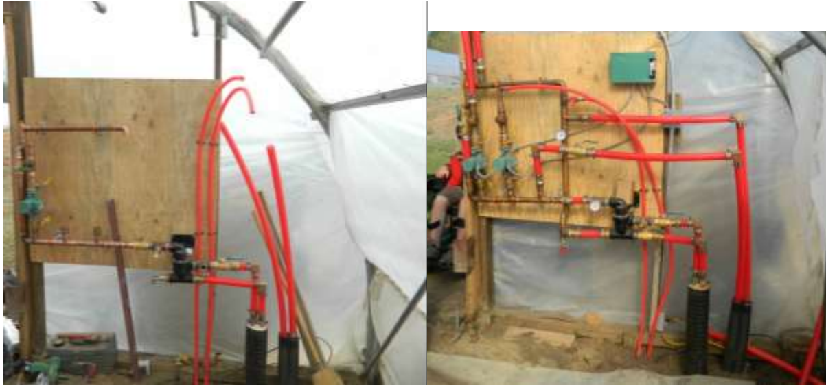
Figure 2 - The photo shows the main manifold being constructed (LEFT) and finished (RIGHT). Note the insulated supply/return PEX (lower right) which is connected to the boiler and (far right) to the south house. This manifold is needed to distribute the hot water to the different forms of heat input used in the two houses.
