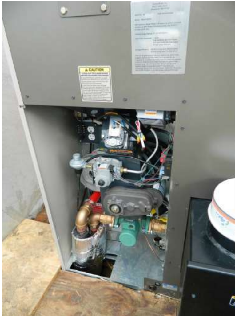
Figure 6 – The water flow to and from the boiler is via insulated underground PEX tubing seen in the lower right corner of this photo. The panel has been removed from the control box to show the propane start/backup burner controls and auger controls. The boiler was plumbed to a main manifold that is in the north greenhouse. From this main manifold the hot water can be sent to (a) an air heater in the north house, (b) in ground heating in the north house, (c) an air heater in the south house, or (d) bench heating mats in the south house. The control of the hot water distribution is both manual (valves) on a seasonal basis and automatic (thermostat) once the sub-system has been enabled for the season.
