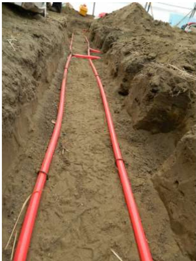
Figure 4 - PEX tubing was buried 12-16" underground in the north house for root-zone heating of tomatoes. Dave has noted a significant boost in early growth as a result of putting heat into the ground near the root zone of this crop.
