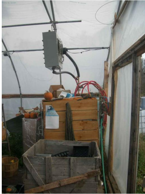
Figure 3 - Homemade insulated hot water tank (beyond the wooden crate) with the other hydronic unit heater overhead.
