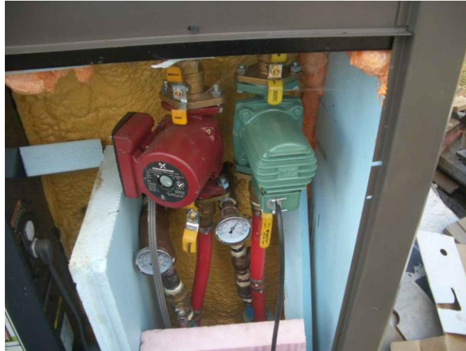
Figure 5 - Circulators mounted on the boiler. Grundfos is red, Taco is green.
