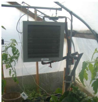
Figure 2 - One of Paul's two hydronic unit heaters. Also note the insulated piping coming out of the ground from the other house.
