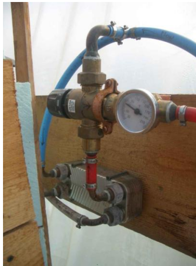
Figure 4 - Water heating system for plant watering.
