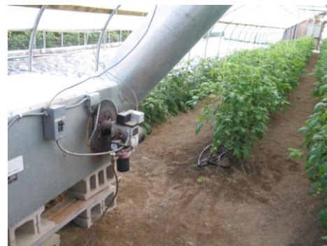
Oil furnace with a Beckett burner inside a tomato greenhouse
