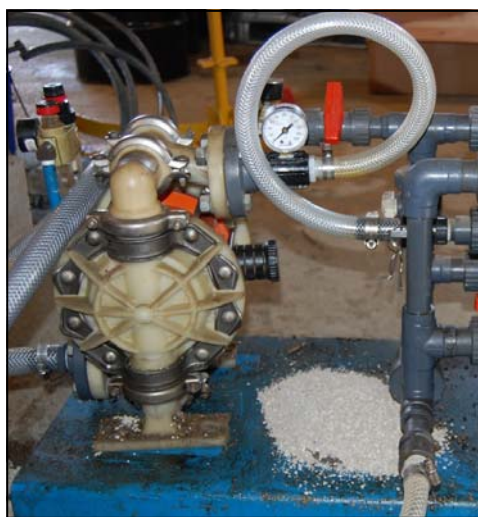
Figure 2.4.10: Air operated diaphragm pump on filter press.
