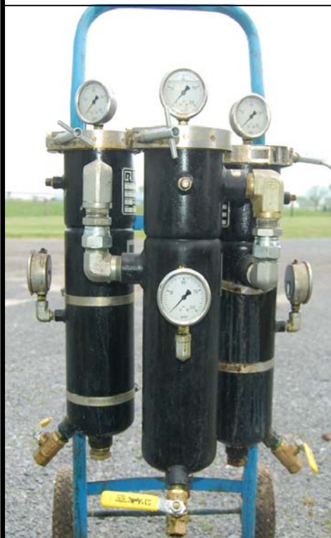
Figure 2.4.4: Three bag filters and housings arranged in series.
