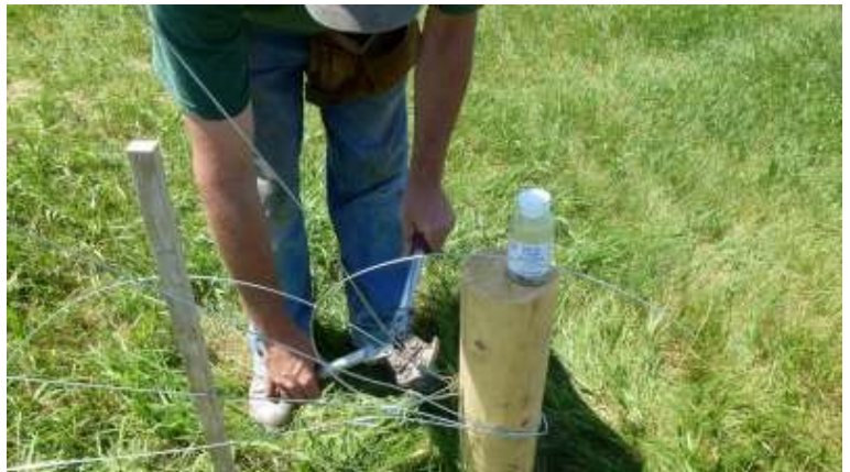
Crimp sleeves and wire crimper/stripper/cutter are used to fasten the tensioned trellis wire
