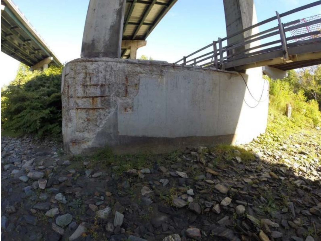
Figure 5.46 End view of pier base with damaged concrete removed on I-89 Waterbury Overpass Bridge
