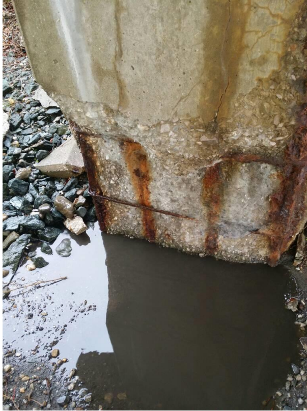
Figure 31: Severe spalling and steel corrosion on column and footing. Notice that some of the steel reinforcement is non-existing.
