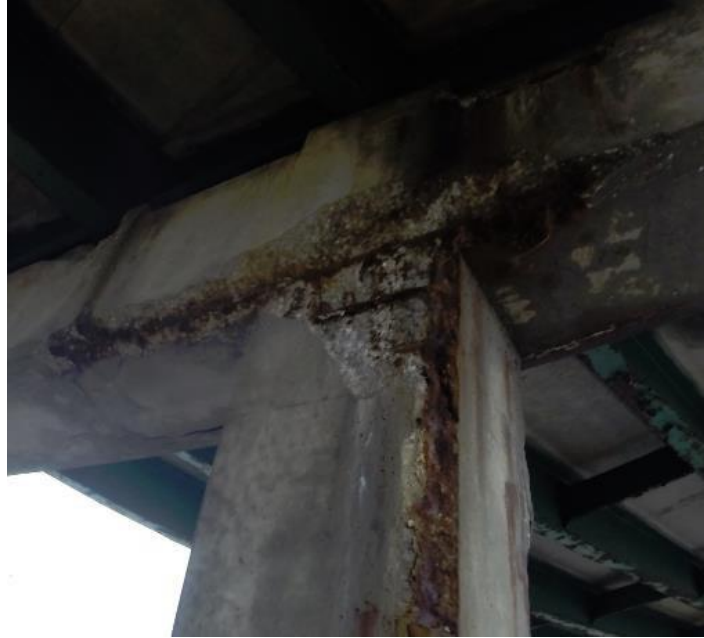
Figure 20: Close-up of concrete spalling and steel corrosion on middle column and cap
