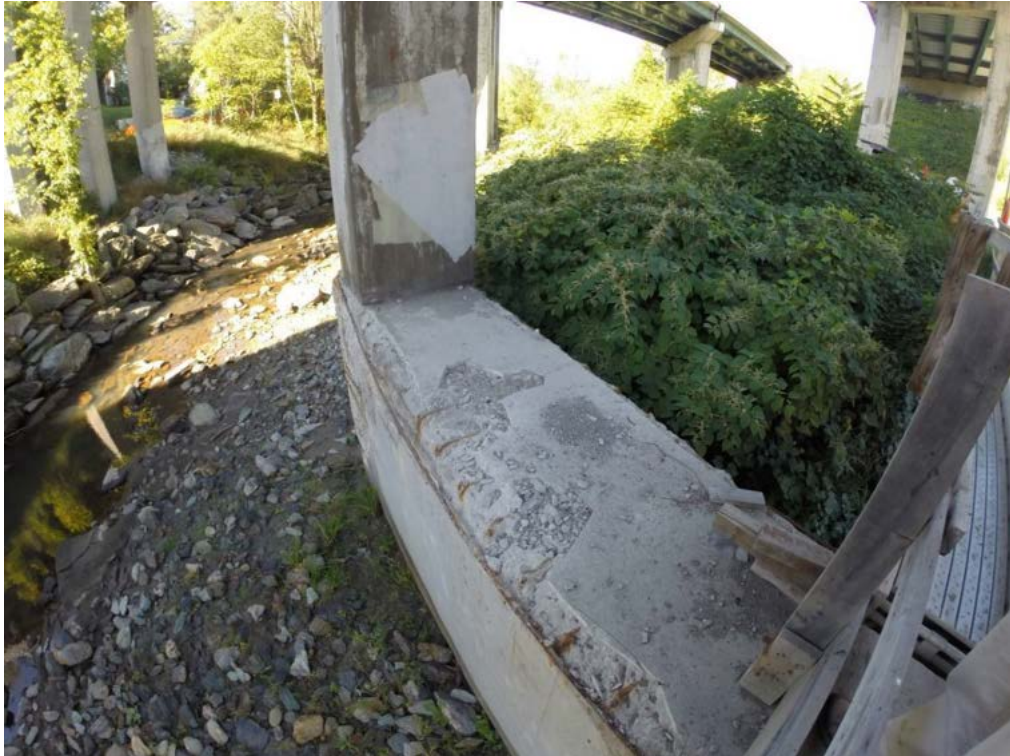
Figure 5.47 Top view of pier base with damaged concrete removed on I-89 Waterbury Overpass Bridge
