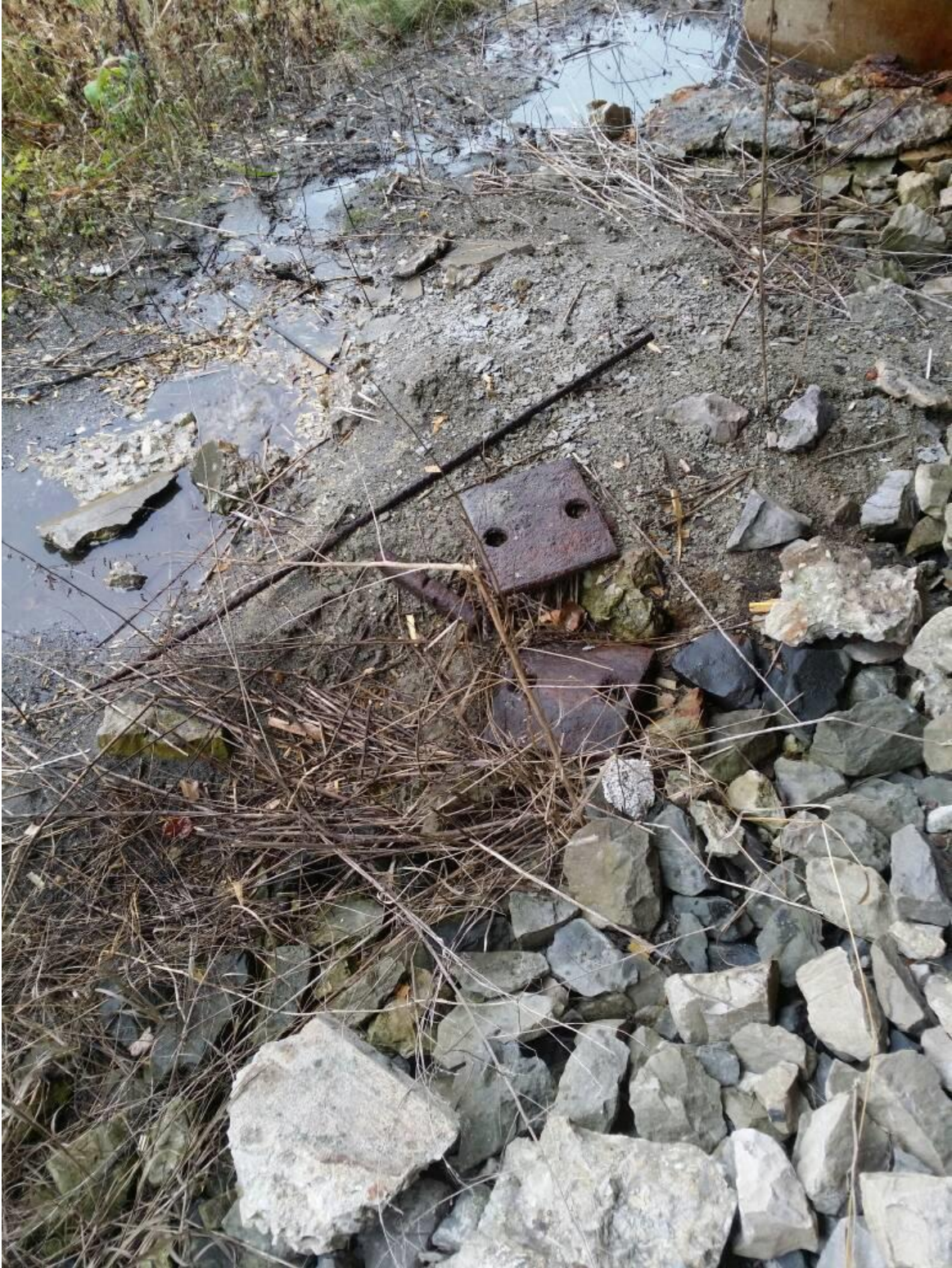
Figure 5.39 Pieces from subsided bearing on Richmond I-89 US 2 Underpass Bridge
