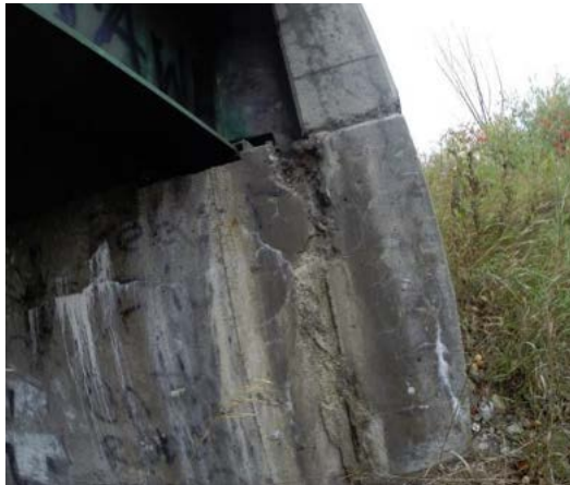
Figure 29: Scaling on abutment around bearing and beam
