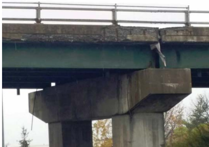
Figure 27: Spalling and steel corrosion on concrete fascia.
