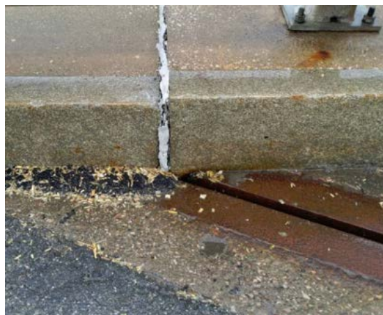
Figure 35: Bridge deck and expansion joint. Because of non-existing bearing bridge deck has settled down about 1.5”.
