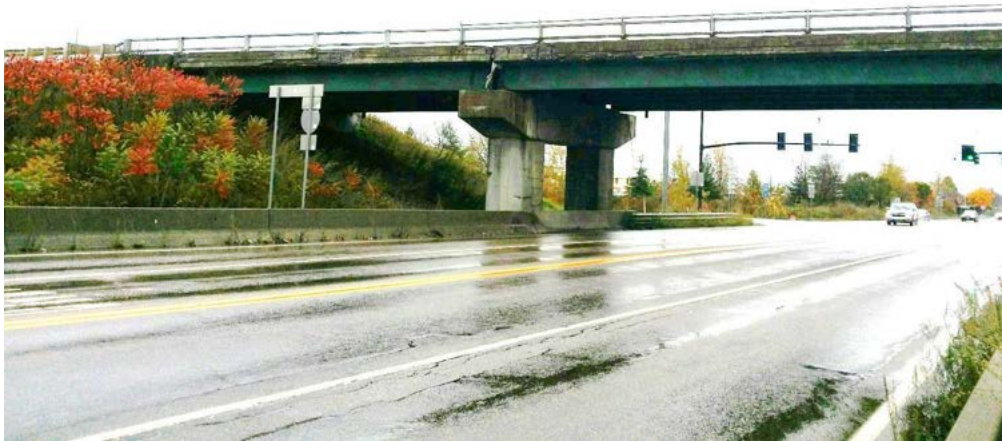
Figure 5.21 Williston I-89 Overpass Tafts Corner with encasement repair of the pier, failed expansion joint gutter and distressed fascia
