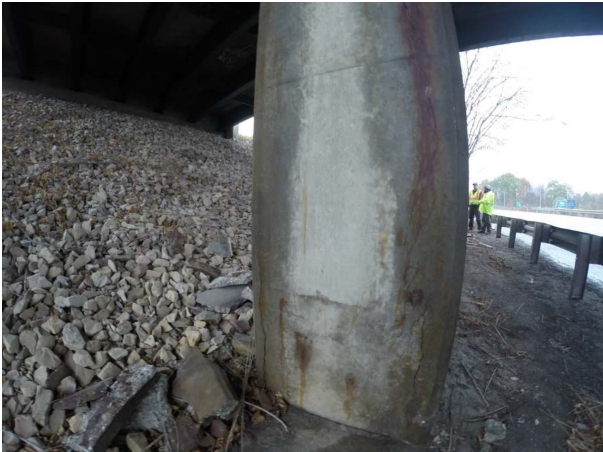
Figure 5.9 Column on Colchester/Milton I-89 Bridge showing cracking, likely due to swelling corroded reinforcing bars
