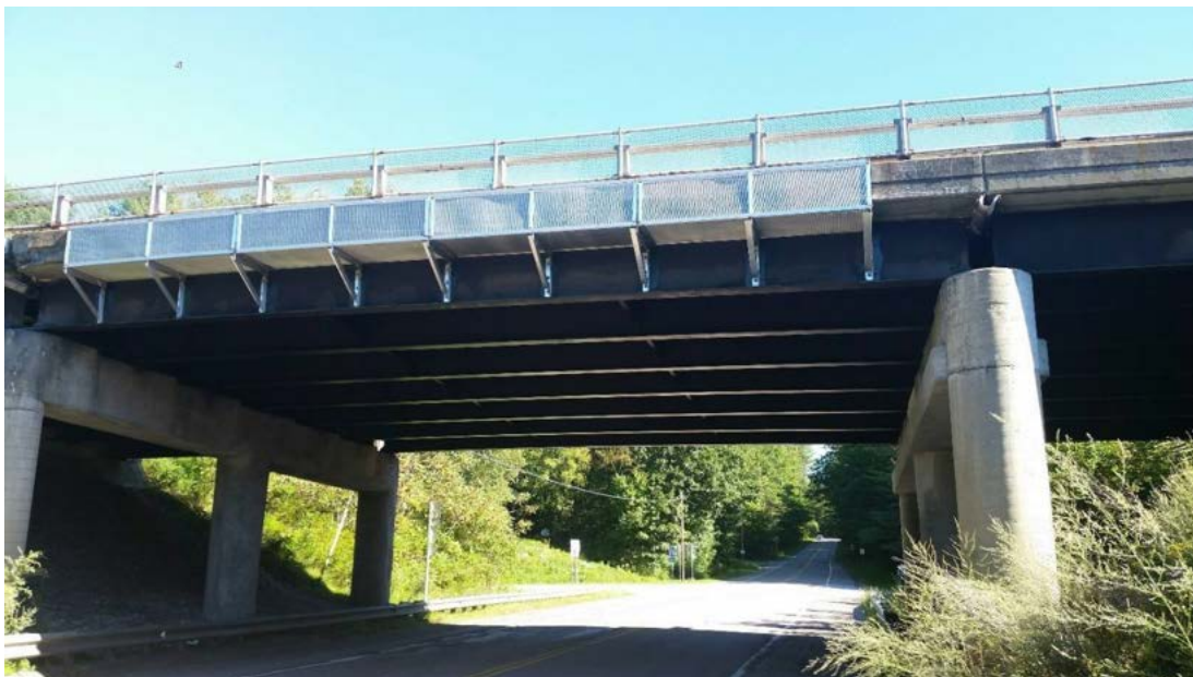
Figure 5.53 I 89 Middlesex Overpass Bridge with supplemental rack to protect vehicles passing under by catching pieces of concrete that spall and fall from the fascia
