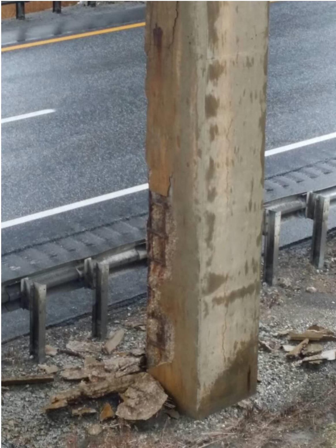
Figure 5.36 Column with spalling at the corners and side on Richmond I 89 US 2 Underpass Bridge
