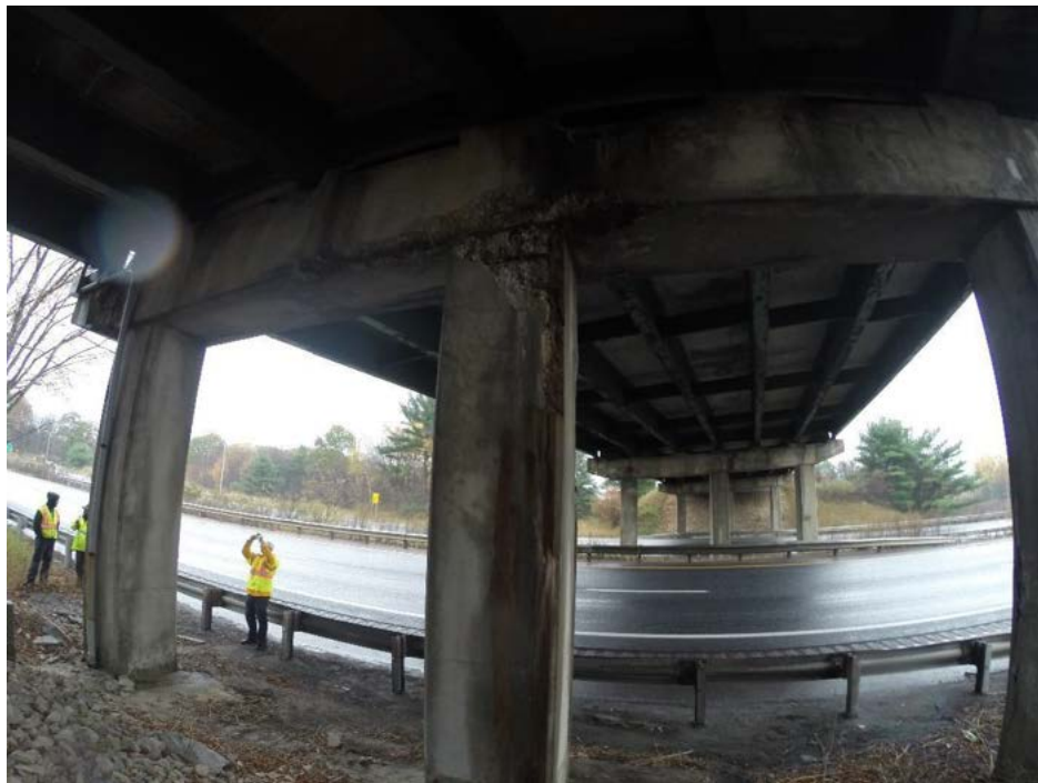
Figure 19: Column and cap Spalling and steel corrosion
