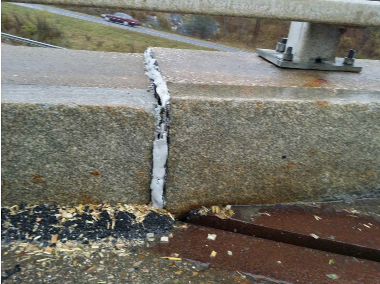
Figure 5.40 Subsided bearing leading to vertical misalignment of expansion joint on Richmond I-89 US 2 Underpass Bridge
