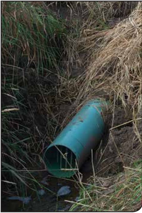
Figure 1: Tile outlet with a rodent guard.
