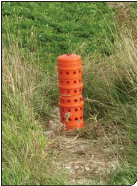
Figure 3: Typical tile vents/surface inlets.
