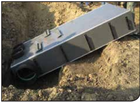
Figure 4. Water level control structure for tile drains
