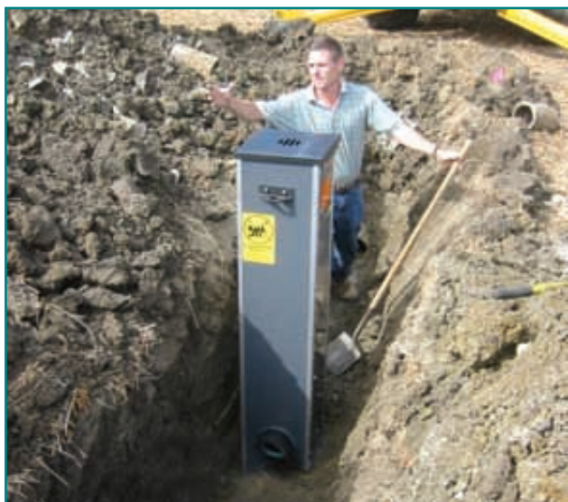
In drainage water management, water control structures are used to vary the depth of the drainage outlet. Flatter fields require fewer structures.
