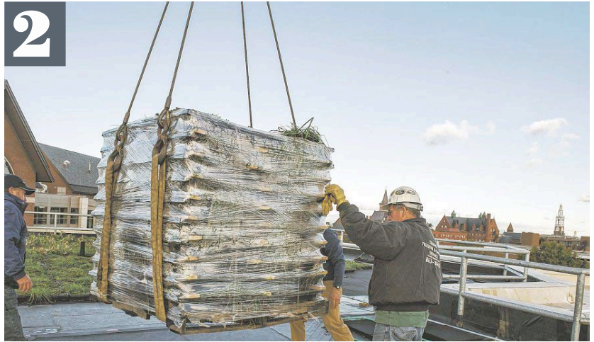
A crane was used to hoist the flats to the roof, which, during the building's renovation, had been molded with insulation by the builders to form the eight separate watersheds.
