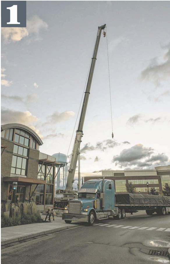
A truck arrives at the Aiken Center on Oct. 11, carrying one delivery of the nearly 875 flats of plants to be installed on the roof.
