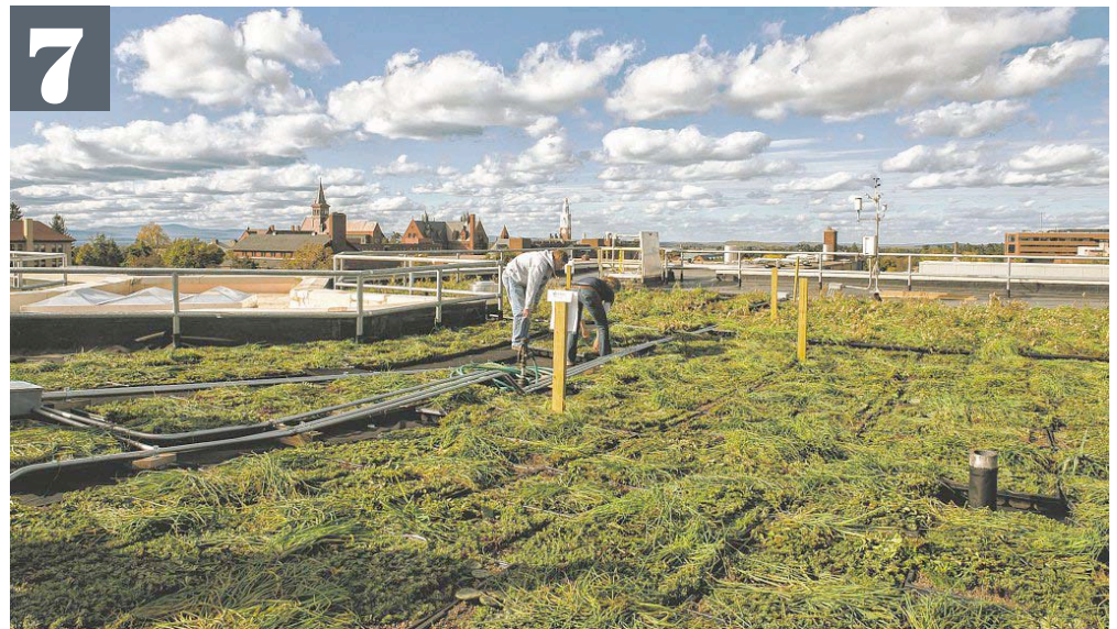
7 Says Hawley, "We just finished putting it in, but now we get to learn from it." Data collected from the roof will be displayed in the building and accessible via the Web.
