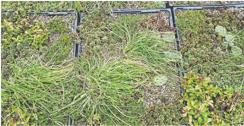
Some of the vegetation making up the green roof at the Aiken Center. GLENN RUSSELL/FREE PRESS
