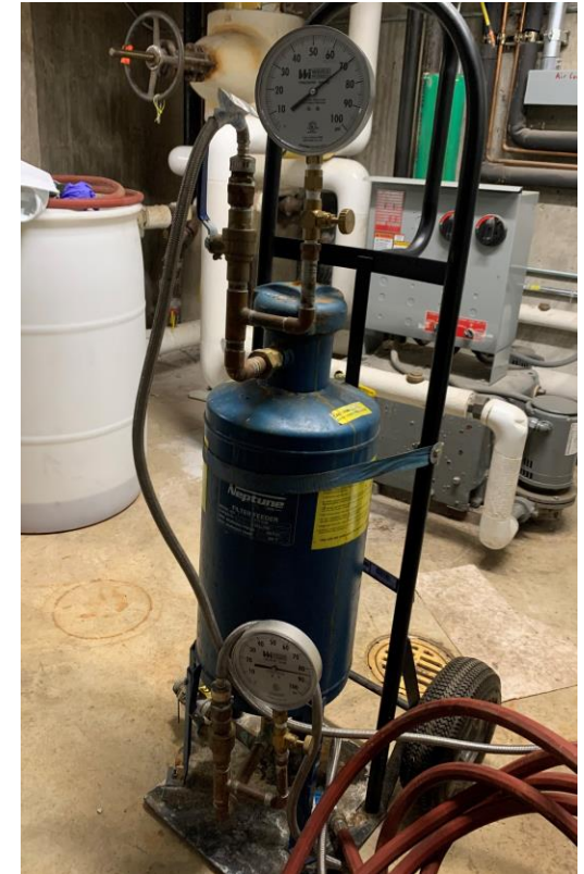
Portable filtering "skid" custom designed for cleaning UVM mechanical equipment
