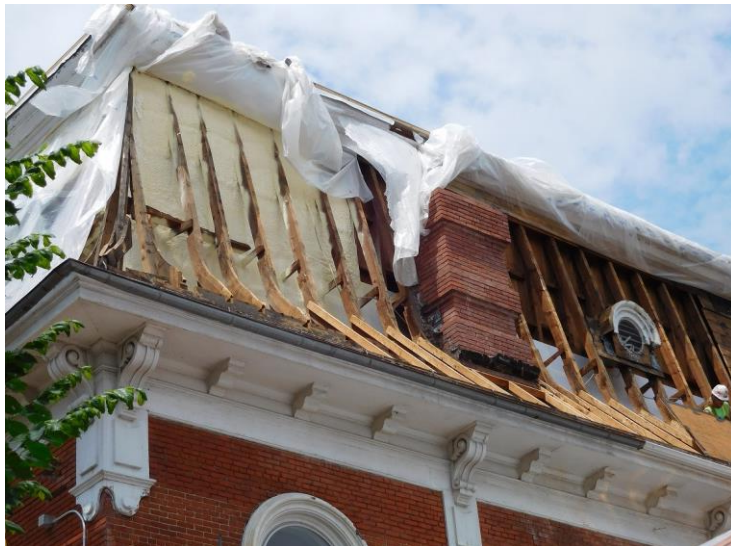
Firewall had been installed just weeks prior to the fire.
