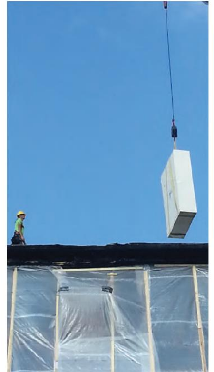
One of the new metal cabinets coming out of the roof of Torrey Hall, day 6 (photo, Sid Bosworth).
