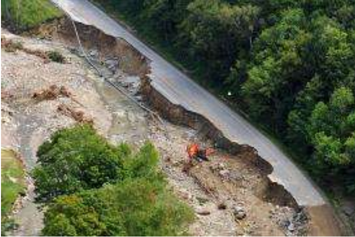
Figure 5: Route 4 near Killington after Tropical Storm Irene. Repairing storm damage may have increased Gross State Product, but did not constitute a positive contribution to our wellbeing.
