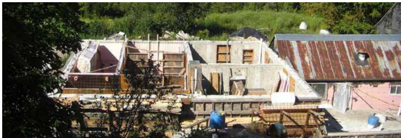
"Butcher Shop Under Construction." Image used with permission of Walter Jeffries. ©2012 Walter Jeffries, SugarMtnFarm.com
