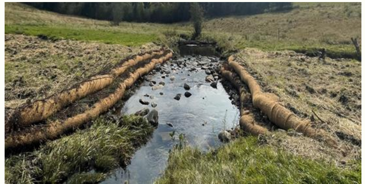
Streambanks & a riffle were constructed where the ski lift tower culvert had been
