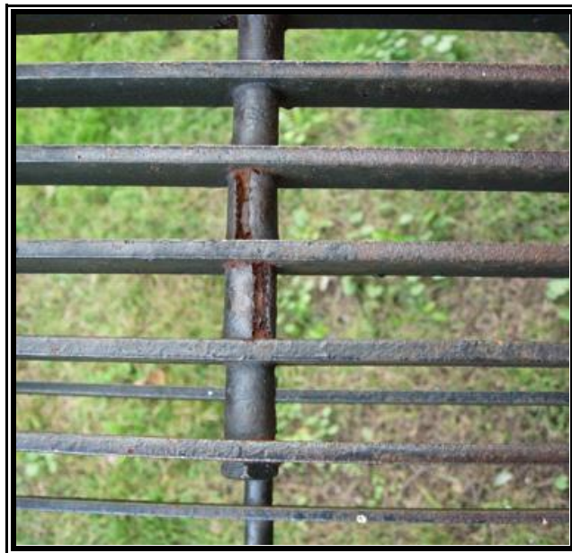
Figure 106: Voids in stair tread need to be filled (author, 2005)
