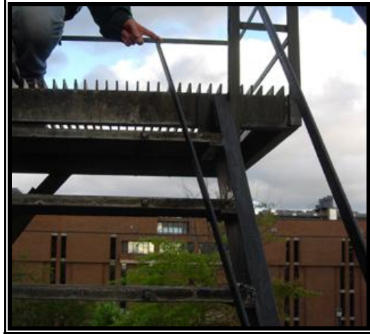
Figure 107: Railing has become detached due to severe oxidation (author, 2005)
