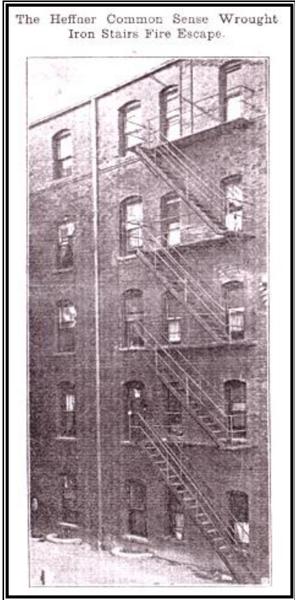
Figure 101: Heffner Common Sense Wrought Iron Stairs Fire Escape (Heffner Iron and Steel Works. The Heffner Fire Escapes . Minneapolis: The Firm, 1901: 2)
