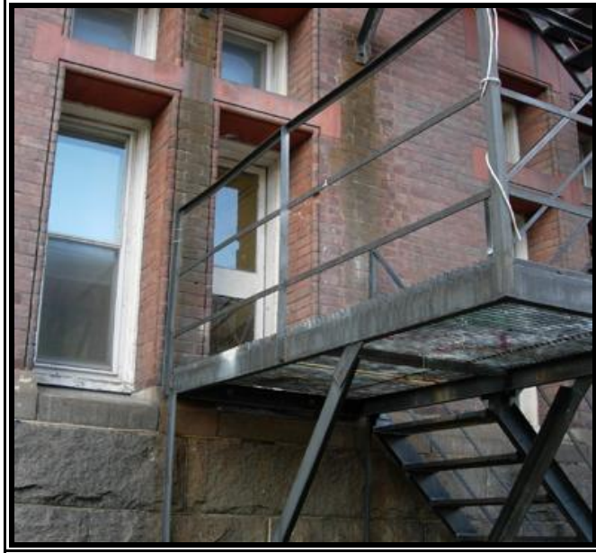
Figure 105: Rust runs down the masonry facade; anchorage many have weakened (author, 2005)
