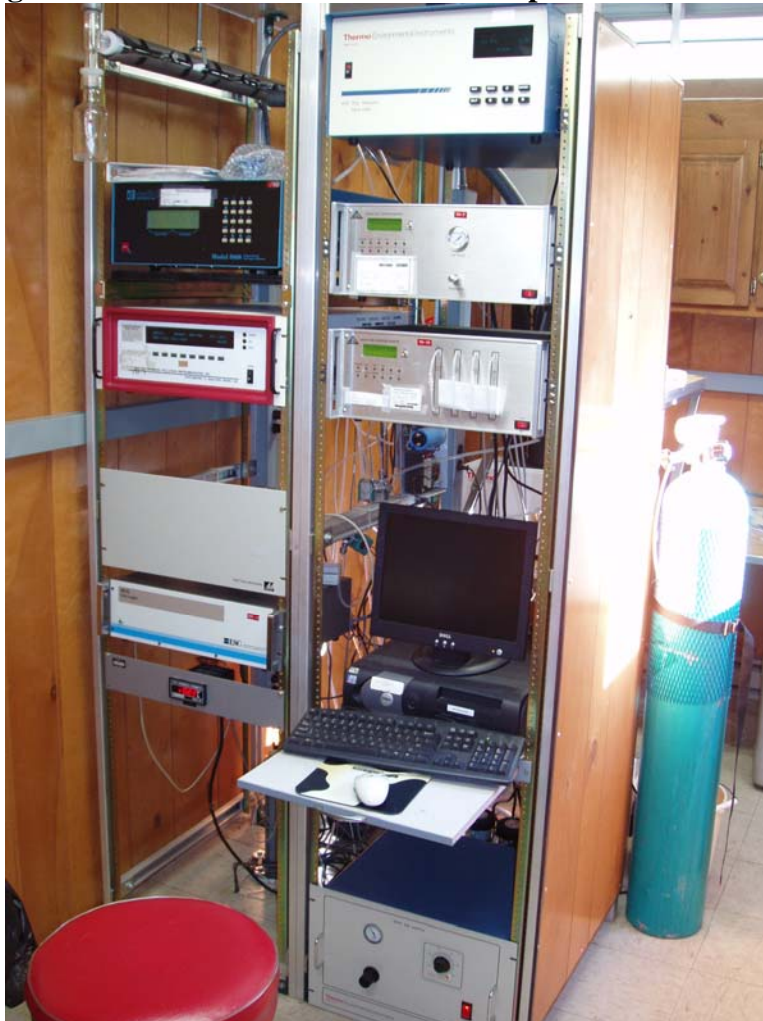
Figure 6 – Current Interior Shelter Setup
