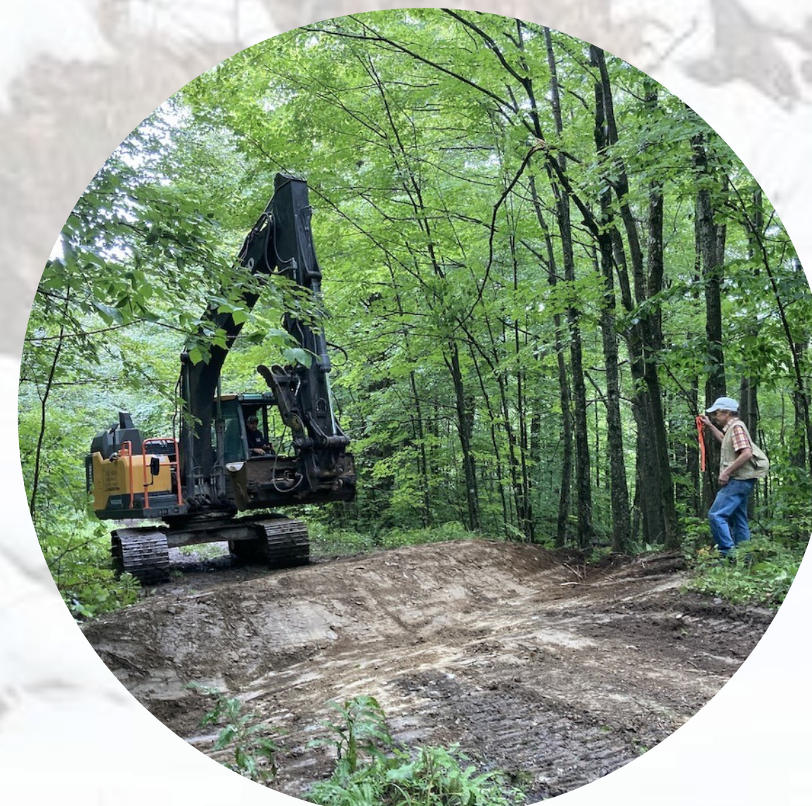
Vermont Family Forests Executive Director David Brynn (right) watches as Chris Cram excavates a broad-based dip on a forest access road.
