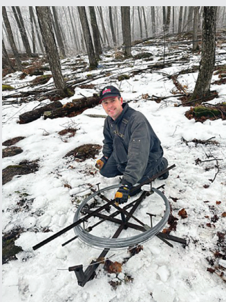
Work underway to remove a dangerous high snag and Scott replacing pipeline after sugarbush thinning
