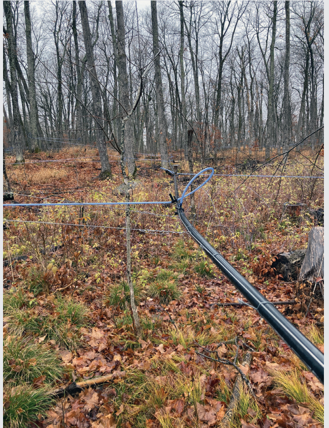
Reconfigured mainline wires in sugarbush
