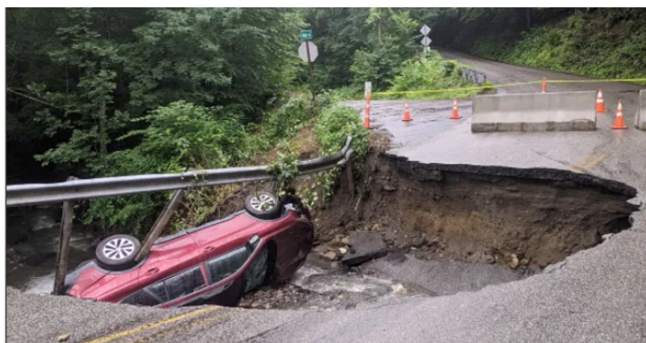
Figure 1 Culvert collapse in a road in Brattleboro, Vermont following heavy rain, 2021 Source: Joshua Carnes (2021)
