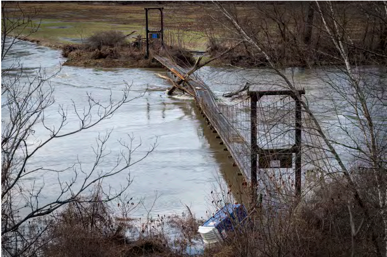
Figure 7-10 Flooding from the Winooski River in Waterbury, Vermont on Dec. 19, 2023
