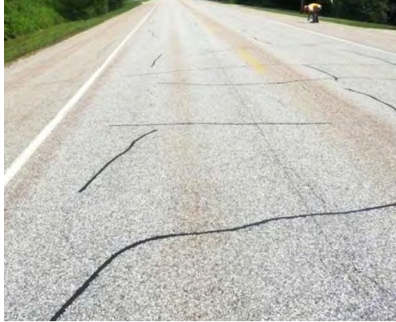
Figure 7-8 Example of a transverse (thermal) cracking of pavement in Dorset, Vermont, 2015
