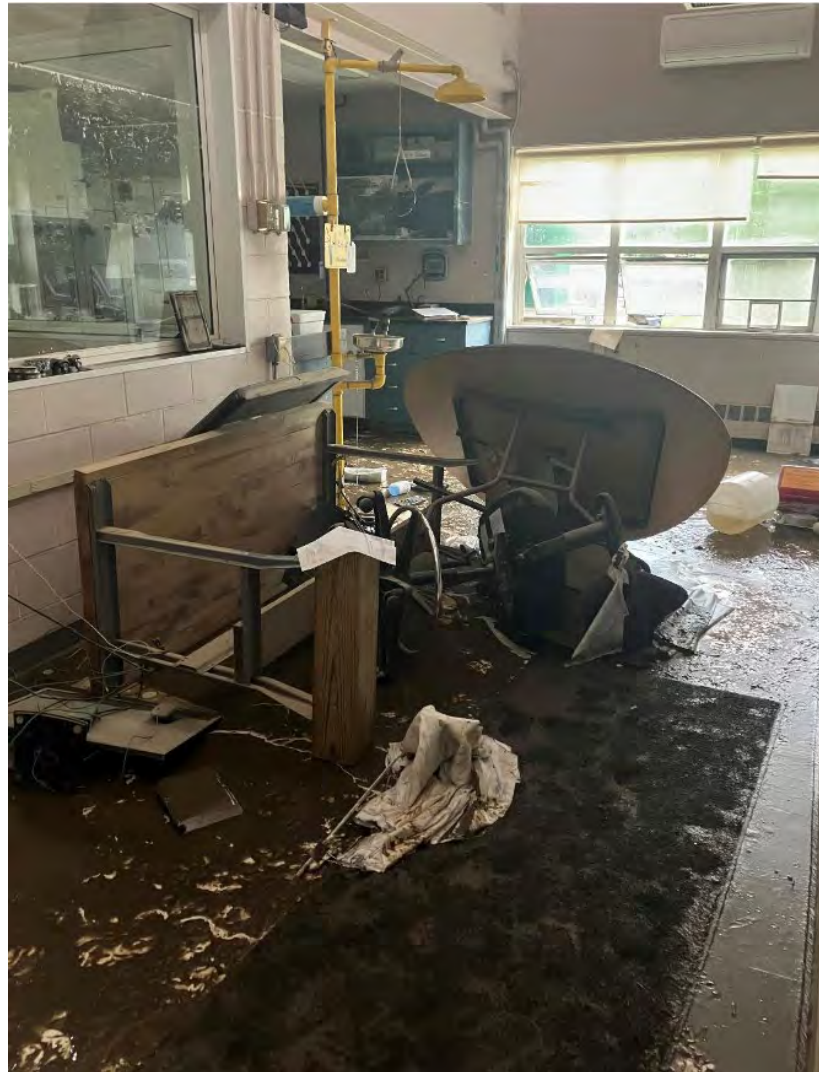
Figure 7-20 Damage to the Johnson Wastewater treatment plant control room after the July 2023 floods. The high-water mark can be seen on the windowpane at the top left corner of the image
