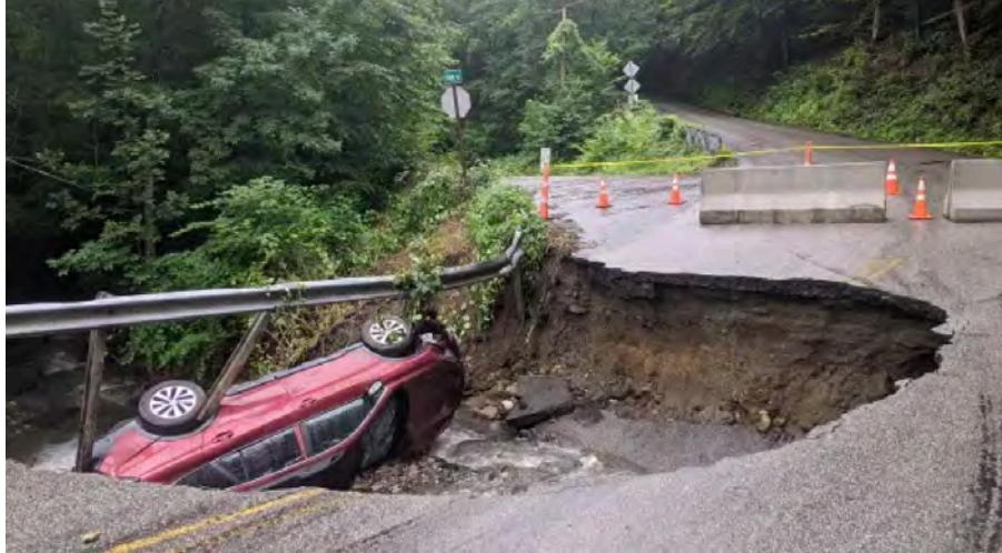
Figure 7-1 Culvert collapse on a road in Brattleboro, Vermont following heavy rain, 2021
