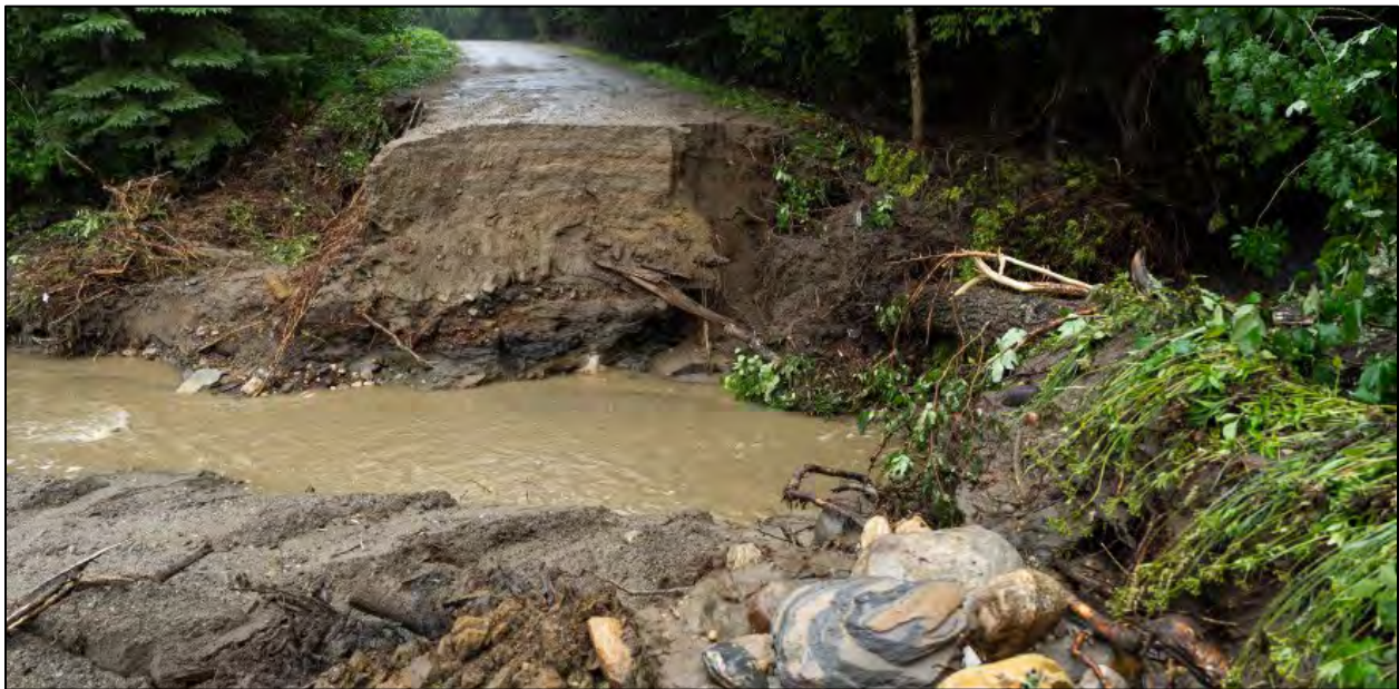
Figure 4-13 Fluvial erosion damage in Addison County from July 2025 flash flooding
