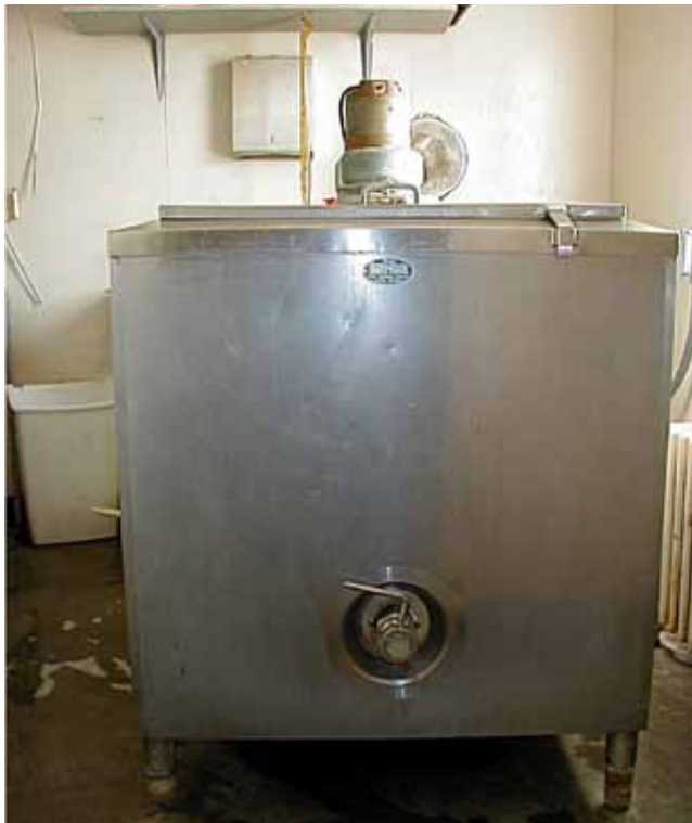
Photo 11.2 100-gallon ice bank bulk tank.
