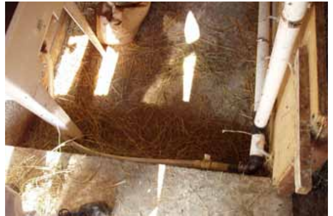
Photo 3.2 A flexible tube with a valve connects the reservoir to a PVC pipe which runs along and is mounted on plywood.
