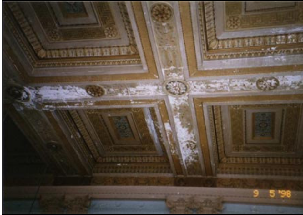
Figure 3.15: Pre-rehabilitation interior photograph taken September 5, 1998, showing deteriorating conditions of the once ornate ceiling in the Lorain Street Savings & Trust's first floor bank lobby. Source: Ohio Historic Preservation Office. (RITC file: 3500 Lorain Avenue, Cleveland, Ohio.)
