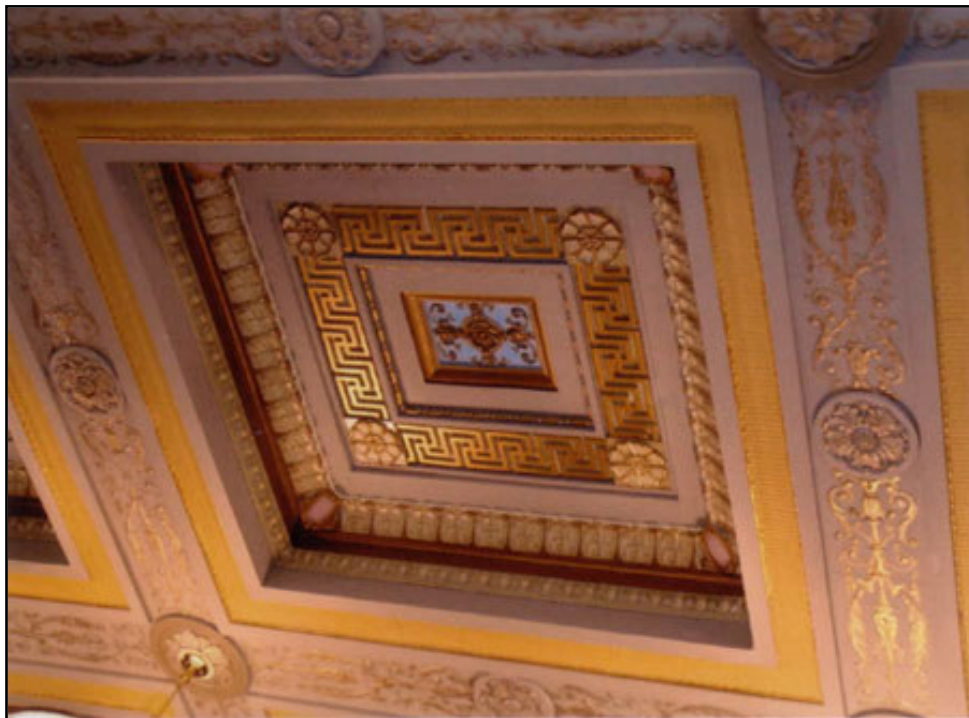
Figure 3.16: Restored ceiling in the first floor bank lobby of the Adam Joseph Lewis Cleveland Environmental Center. Circa 2006. Source: Ohio Historic Preservation Office. (RITC file: 3500 Lorain Avenue, Cleveland, Ohio.)
