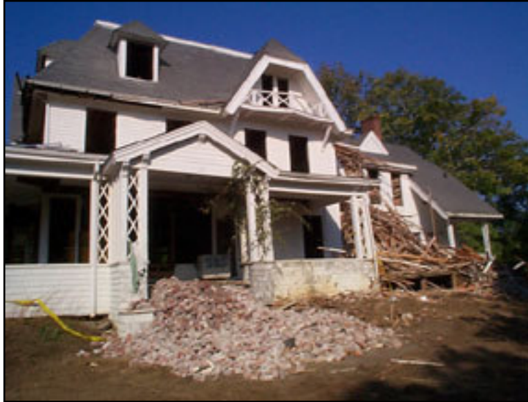
Figure 2.17: The Gilman Ordway Campus project involved demolition and removal of significant architectural features, including the Helen Turner House's historic hipped roof, rear wing, brick chimneys, and windows. View looking west. Fall 2001. Courtesy of Woods Hole Research Center.
