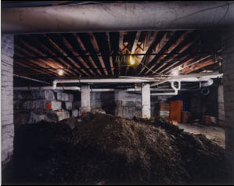
Figure 4.7: Photograph of Trinity Church’s unfinished basement before rehabilitation. Circa 2002. Photograph © Peter Vanderwarker. Courtesy of Trinity Church in the City of Boston. Used with permission.
