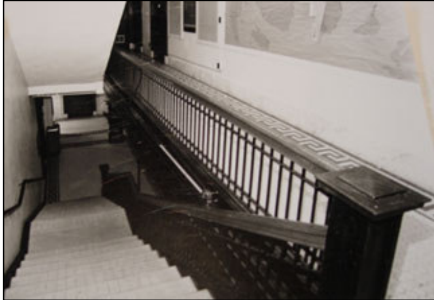
Figure 2.11: Pre-rehabilitation documentation photograph of Barney Memorial Hall interior, showing historic stairs, banisters, and tile flooring. Circa 1997. Courtesy of HRJL Architects, Inc.
