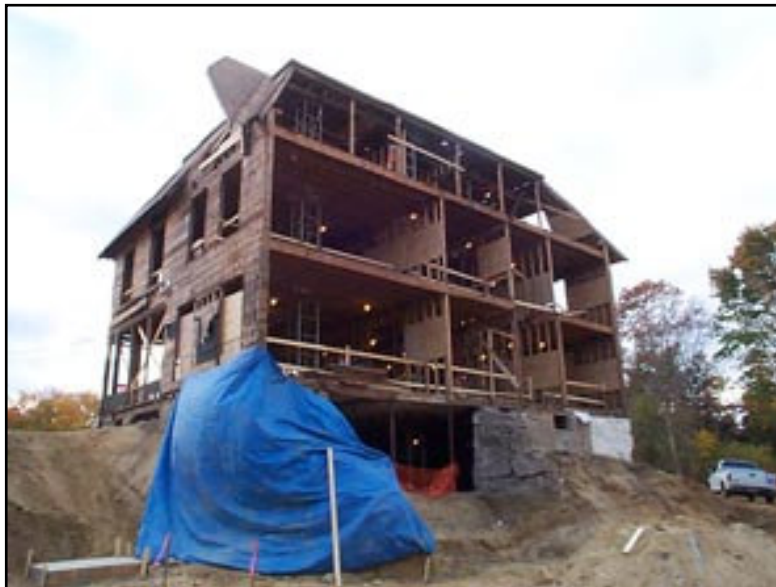
Figure 2.18: The Helen Turner House's historic interior was gutted during the Gilman Ordway Campus project, resulting in the loss of historic fabric and floor configurations. View looking southeast. Fall 2001. Courtesy of Woods Hole Research Center.
