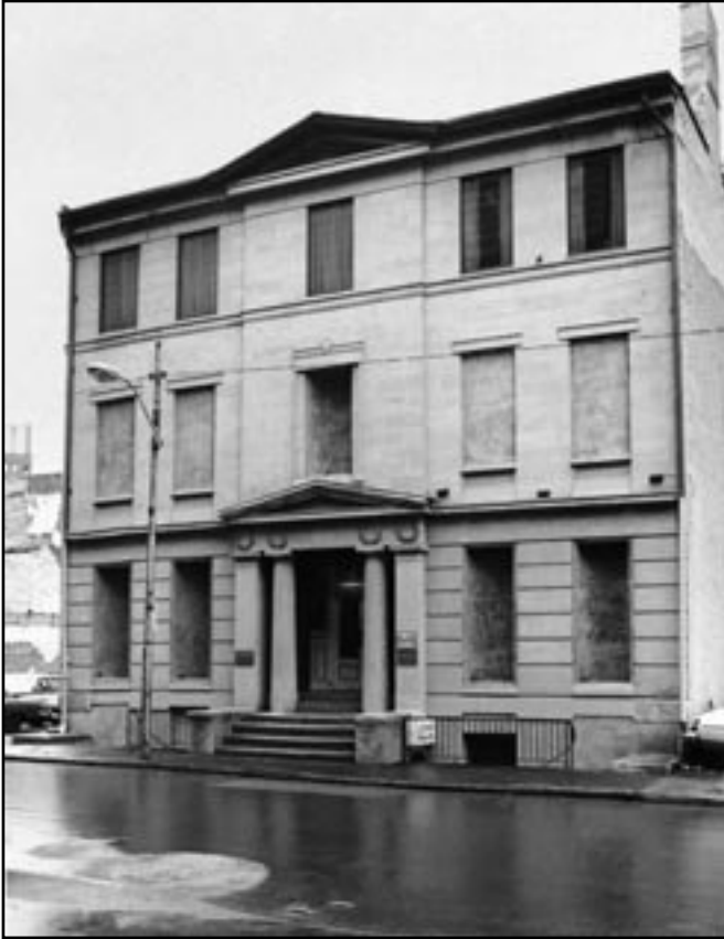
Figure 2.5: Burke Building, circa 1975, in downtown Pittsburgh, Pa. View looking northeast. Source: Allegheny Conference on Community Development Collection, Library and Archives Division Archives, Historical Society of Western Pennsylvania, Pittsburgh, Pa. (Historic Pittsburgh Images Collections, http://images.library.pitt.edu ; item MSP285.B002.F24.I06.) Used with permission of Historical Society of Western Pennsylvania.
