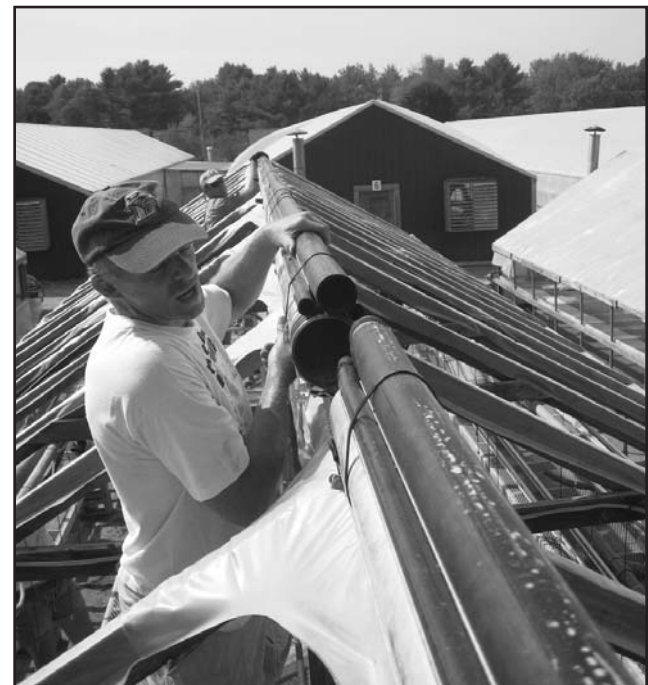
Figure 4. Installation of bubble system by consulting engineer and UVM personnel. Photos by Margaret Skinner
