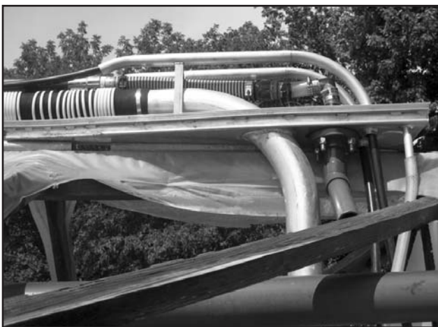
Figure 3. Piping system developed by Sunarc to inject soap bubbles between the two layers of plastic.
