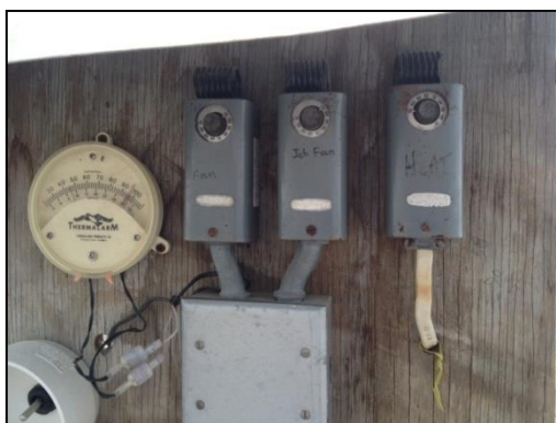
Fig. 18. Older thermostats that should be cleaned annually.
