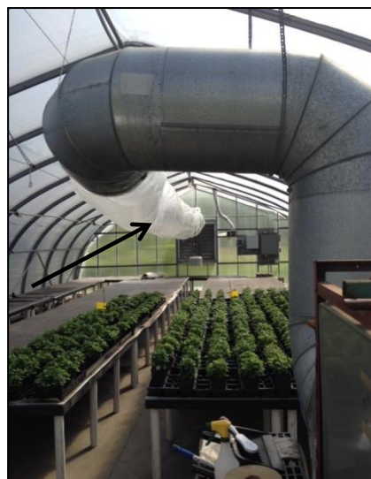
Fig. 19. An overhead heat system that would be more efficient if re-located under the benches. It should be noted that under-bench locations may require increased need for watering.
