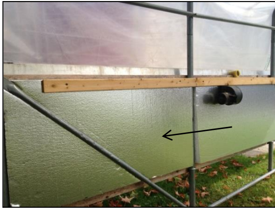
Fig. 5. Aluminum-faced foam board to insulate the end and side walls eliminates the need for the poly layer.
