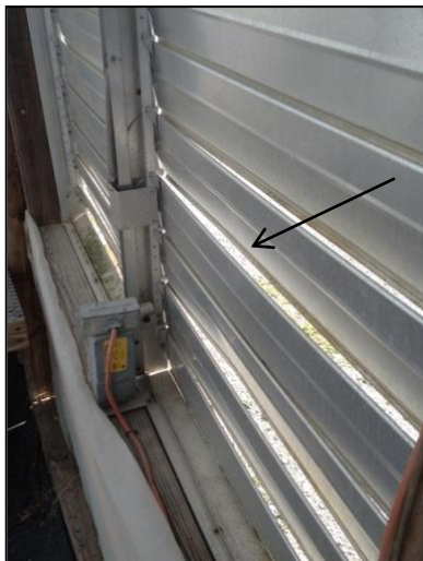
Fig. 7. Improperly adjusted louvers. Note the cracks (indicated with arrow) where heat can easily leak to the outside.
