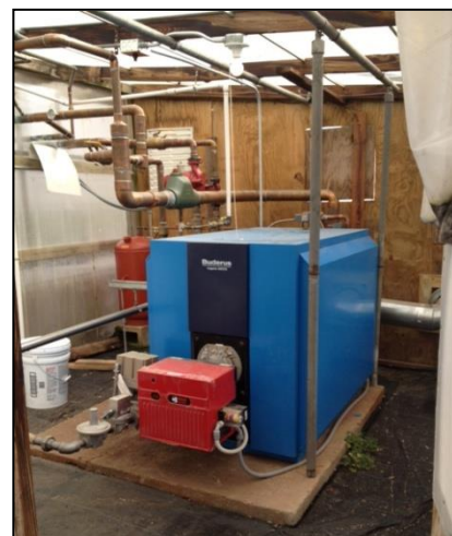
Fig. 16. High efficiency gas furnace.
