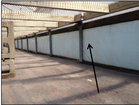
Fig. 9. Foam board insulation on a kneewall from the floor up to bench height covered with poly. Use of aluminum-faced board may eliminate need for the additional layer of poly.
