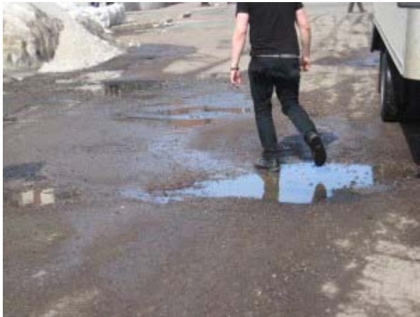
Figure 4: Some of the potholes facing drivers in Chittenden County [Photo credit: Burlington Free Press]
