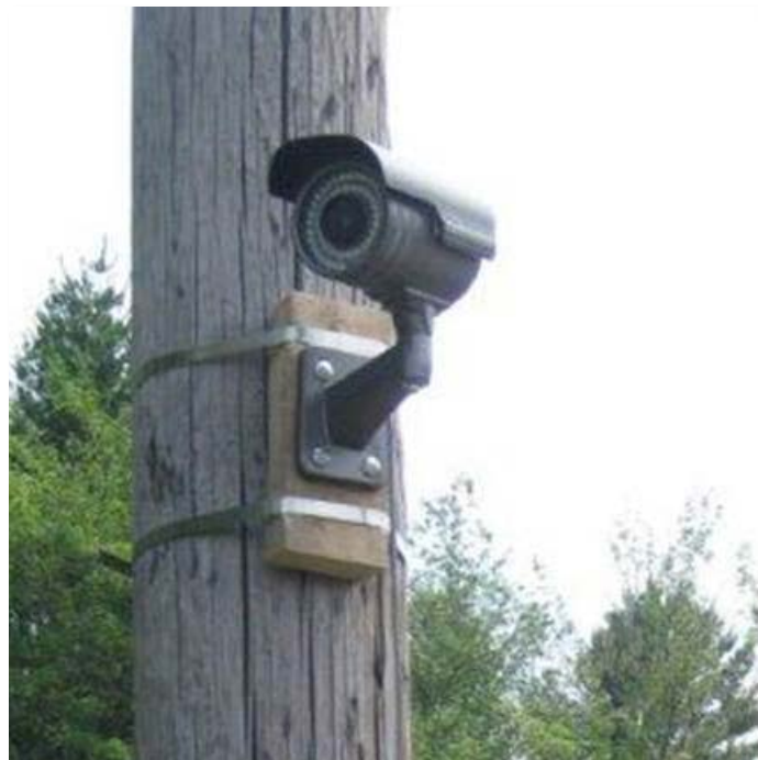
Figure 4 Camera Mounted to Roadside Power Pole
