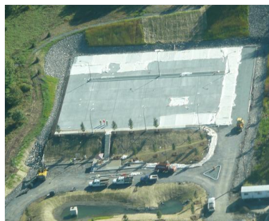
Porous concrete park and ride facility in Randolph, VT: during construction (left), typical cross-section (right), aerial view (below)
