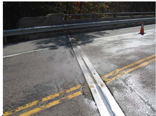
Figure 15. Sealant in the Rhode Island Bridge Joint
