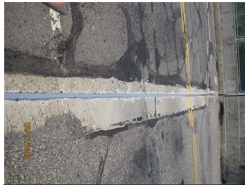
Figure 6. Sealant in the Connecticut Bridge Joint
