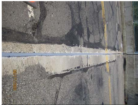
Figure 6. Sealant in the Connecticut Bridge Joint
