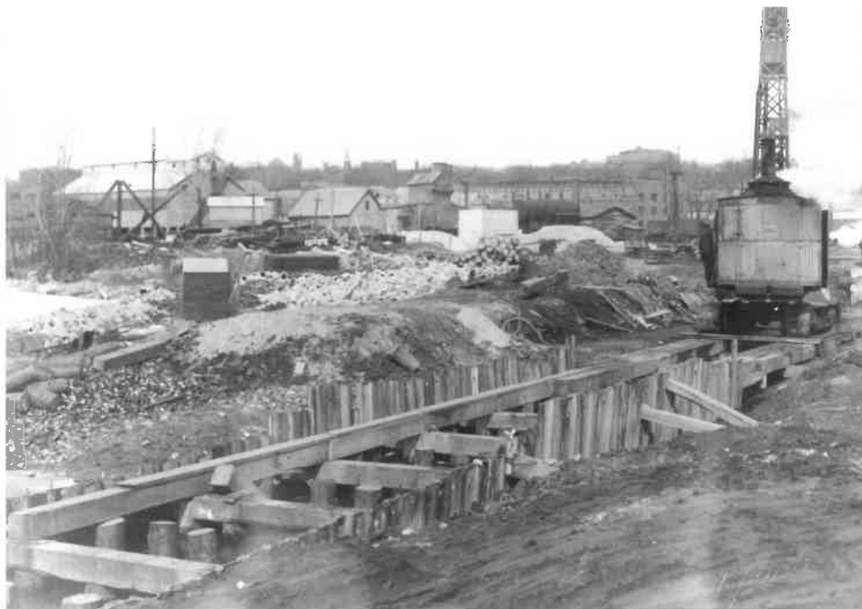
Fig. 11 This 1932 photo, taken during the construction of the main trunkline sewer, looking northeast, gives an idea of the amounts and types of debris found in the fill on the site. On the far left, a heap of old tin cans is visible along with pieces of wood and piles of sewer pipe. (Source: McAllister Photo Collection, Wilbur Special Collections, Bailey-Howe Library, Burlington, Vermont, 1932.)
