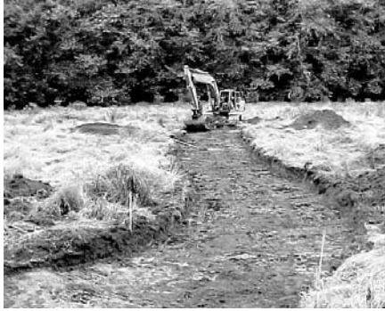
Figure 3. Construction of the new Karnowsky Creek channel, summer 2002. Stakes in foreground identify the location of a transition from a riffle to a pool. Note the excavated mounds of soil left on the floodplain.
