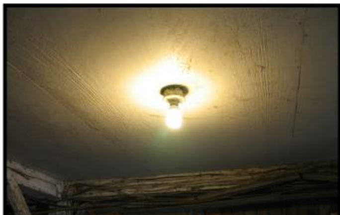
One of 32 lights in the Harlow packing house. if this breaks, glass could fall into produce.
