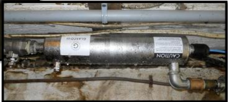
This $1,200 (installed) UV filter kills soil bacteria, making spring water potable
