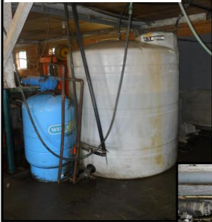
This 1,000 gallon cistern and pressure tank supply water at Harlow Farm
