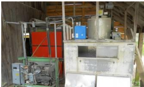
Ice maker compressor and hydrocooler (orange box behind) under a shed roof at Harlow Farm
