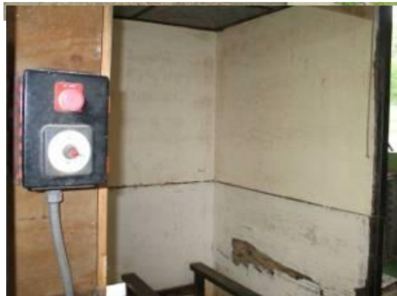
Inner walls of the hydrocooler need patching and smoothing
