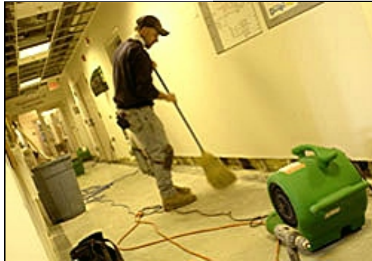
Workers scrambled to dry Old Mill after a split sprinkler dumped freezing water through the fifth and fourth floors. (Photo: Bill DiLillo)
