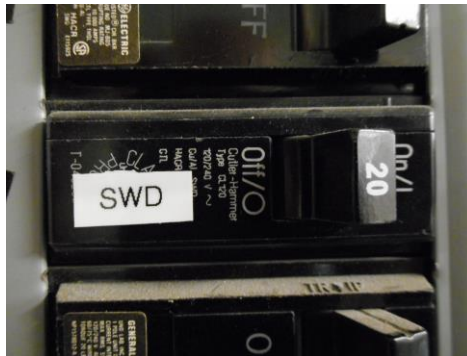
Example : Switch Rated Electrical Circuit Breaker labeled “SWD”
