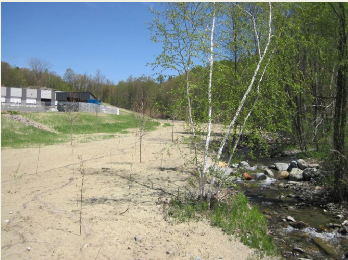
Before (top) & after (below) Beecher Hill Brook floodplain restoration by Lewis Creek Association. Project restored 1.3 acres of floodplain
