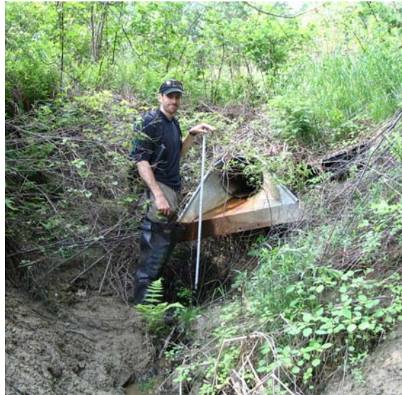
Evan measuring erosion from storm drain pipe in Centennial Brook watershed.
