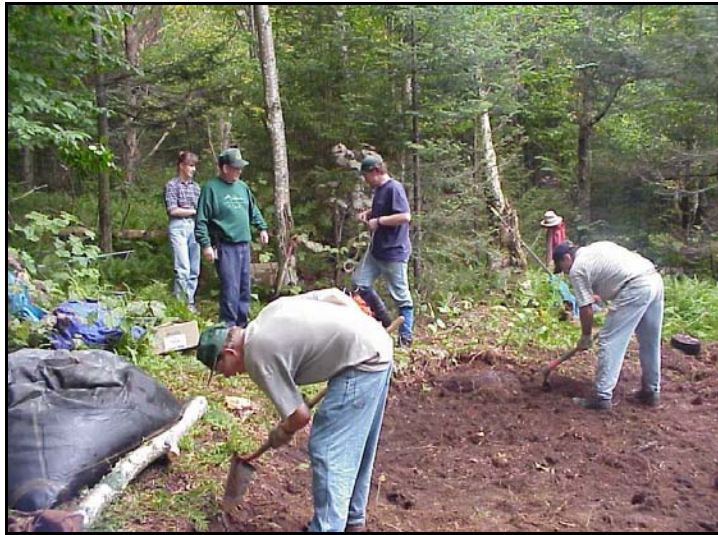
Staff with Vermont Agency of Natural Resources, USDA Forest Service, and USDA Natural Resources Conservation Service help to install snow pillow at Mt. Mansfield SCAN site.
